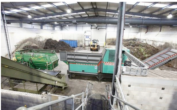
In Vessel Composting - Manchester
